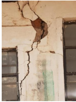
Plate IV: Image of running crack lines showing part of the block work at the Department of Fine Art annex (ABU, Main Campus). Photograph: Zumnan Moses Sekuk (2023)
