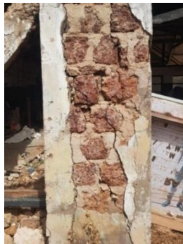
Plate V: Image of EXPOSED stone work as a result of cracked plaster due to heat from a fire outbreak, at the Department of Fine Arts annex (ABU, Main Campus) Photograph: ZumnanMoses Sekuk (2023)
