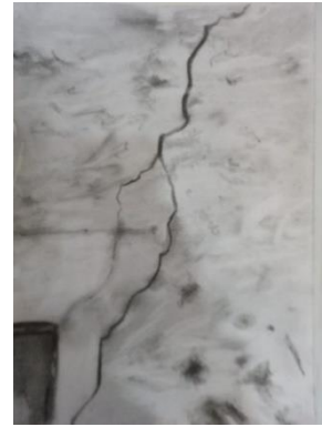
Plate IX: Preliminary drawing of a splitting diagonal crack on a wall, showing apportion of the block work, 21 x 29cm, Photograph: Zumnan Moses Sekuk (2023)
